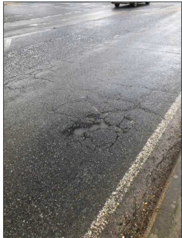
Figure 3-5 - Pothole in Section 1
