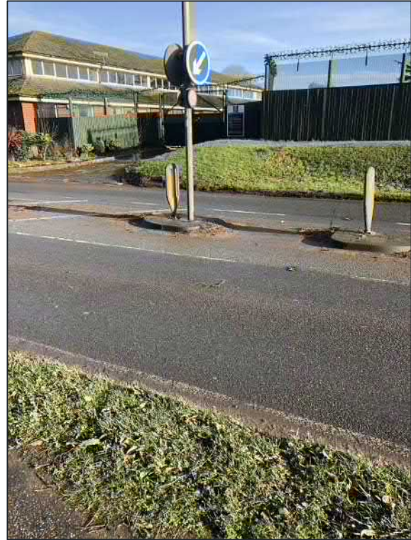
Figure 3-7 - Crossing with no dropped kerb, reducing road width, Section 1
