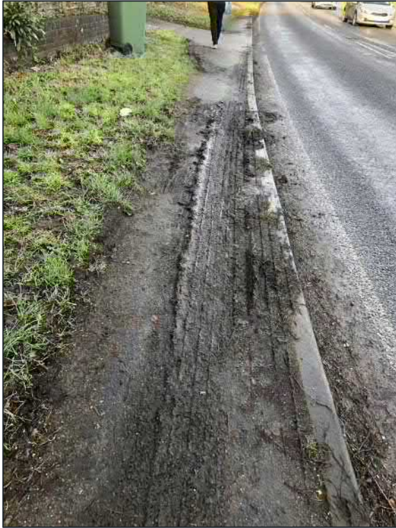
Figure 3-6 - Muddy conditions / cars mounting footway, Section 1
